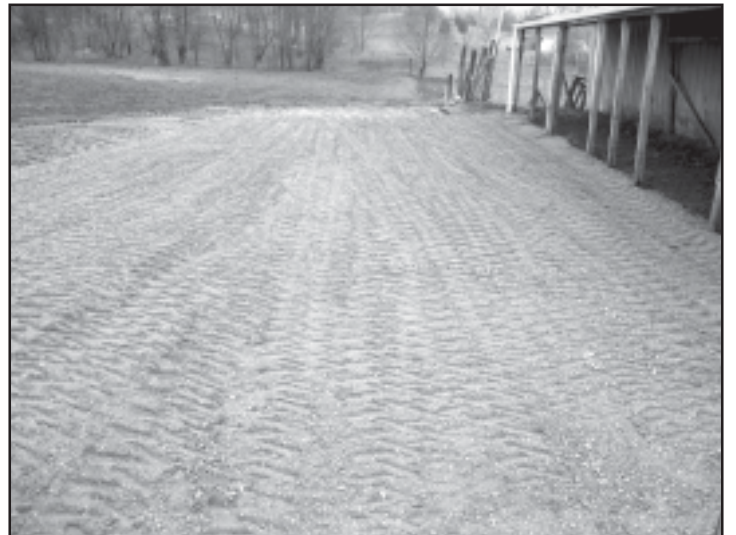
Manure was scraped off of site, #60 Geo cloth was laid and covered with 5" of compacted stone.
